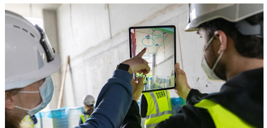
Direct overlay of the planning models with the real building (Gamma AR)
